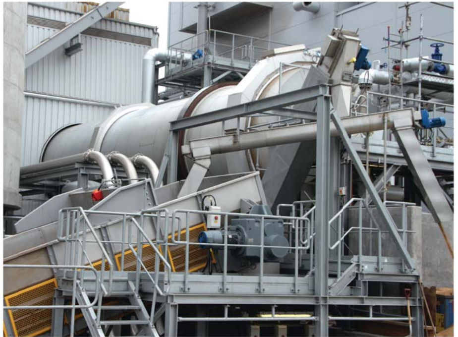
A compact plant, a view of the draff receiving bunker as seen from the side and the rotary steam dryer.
